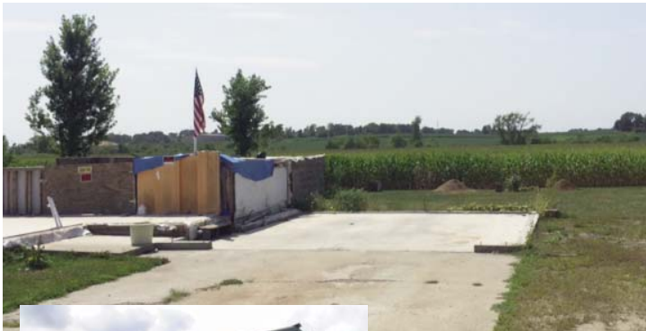
Construction has begun on the community septic tank field (adjacent farm property) which is scheduled for completion by November 1, 2015.
