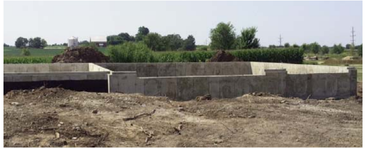
As of August 10, three new foundations are underway in Fairdale, and one in rural DeKalb County. The LTRC estimates that seven more foundations will be dug in the next few months. In addition, five owners are completing the rehabilitation of their homes.
